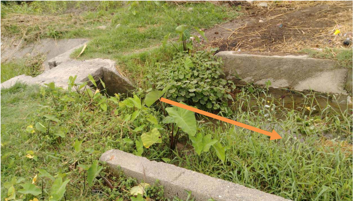
Pic.5: S10-T4, (Ch. 0+093), about 20 cm depth of silt deposited and vegetation growth at u/s and d/s side of DP1
