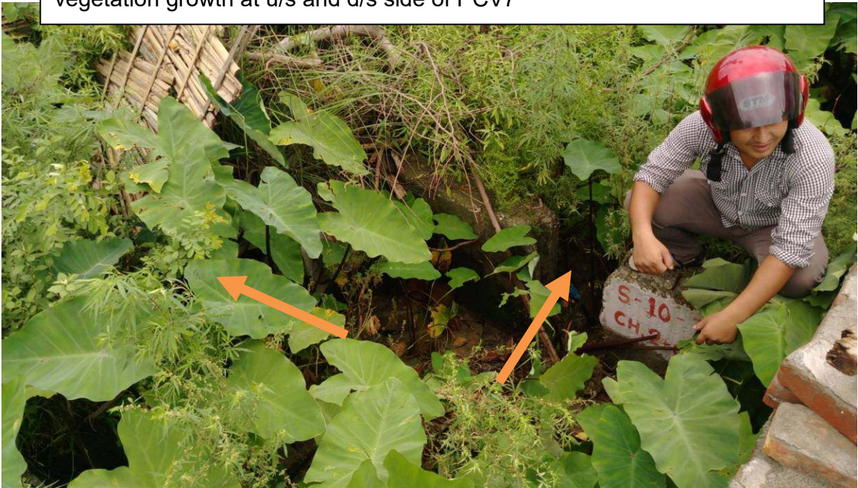
Pic.14: S10-T4, (Ch. 2+614), totally damaged TS
