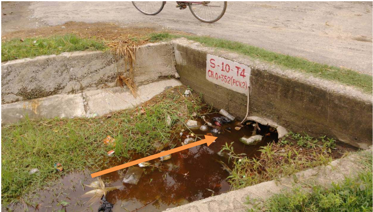
Pic.7: S10: S10-T4, (Ch. 0+353), about 2/3 part of the PCV2 opening is blocked due to siltation, vegetation growth and debris deposition at u/s and d/s side of PCV2
