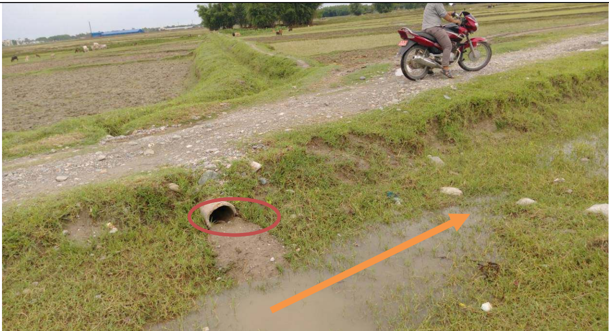
Pic.8: S10-T4, (Ch. 0+650), Masonry structure of WC3L is damaged
