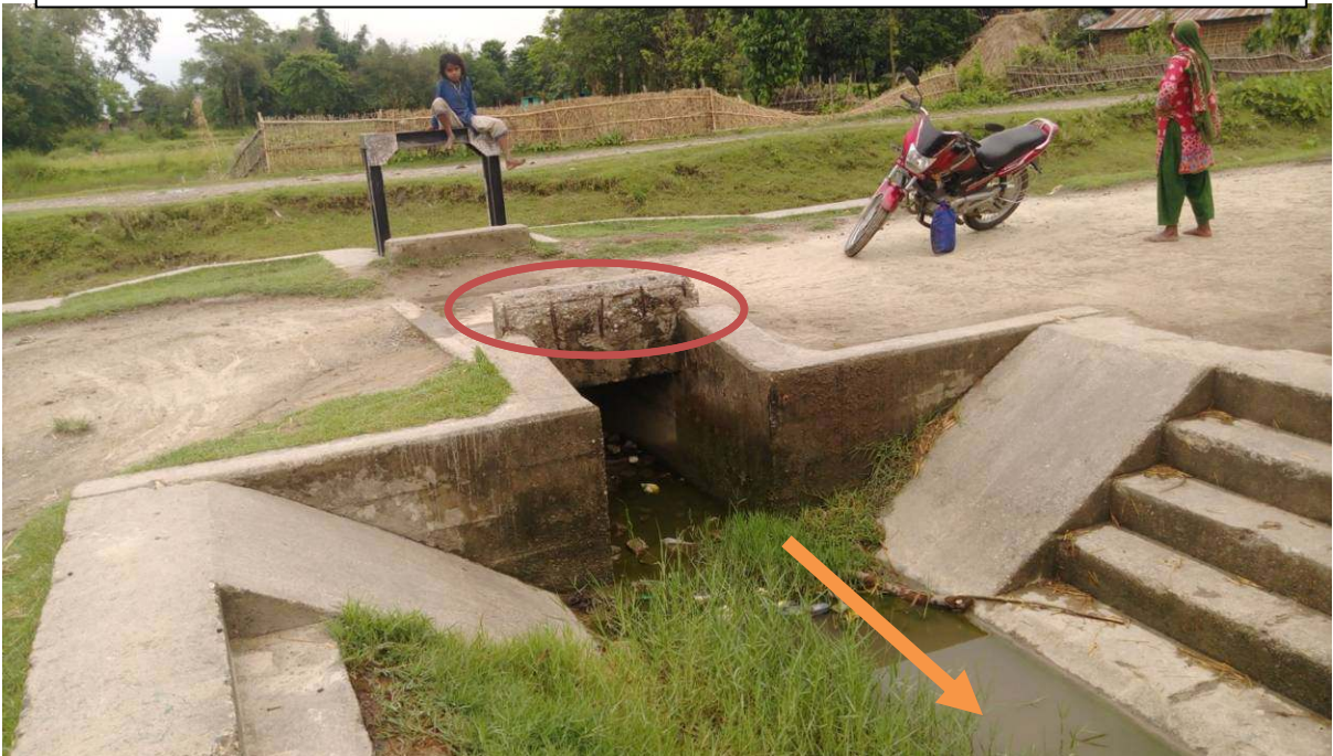
Pic.2: S10-T4, (Ch.0+000), Spalling on d/s side of CV1
