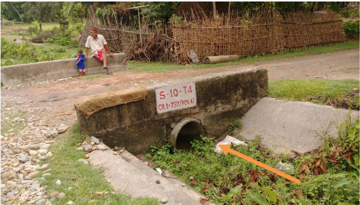
Pic.12: S10-T4, (Ch. 1+753), about 10 cm depth of silt deposited and vegetation growth at u/s and d/s side of PCV4
