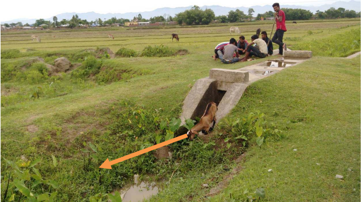
Pic.10: S10-T4, (Ch. 0+881), about 20 cm depth of silt deposited and vegetation growth at d/s side of CV1
