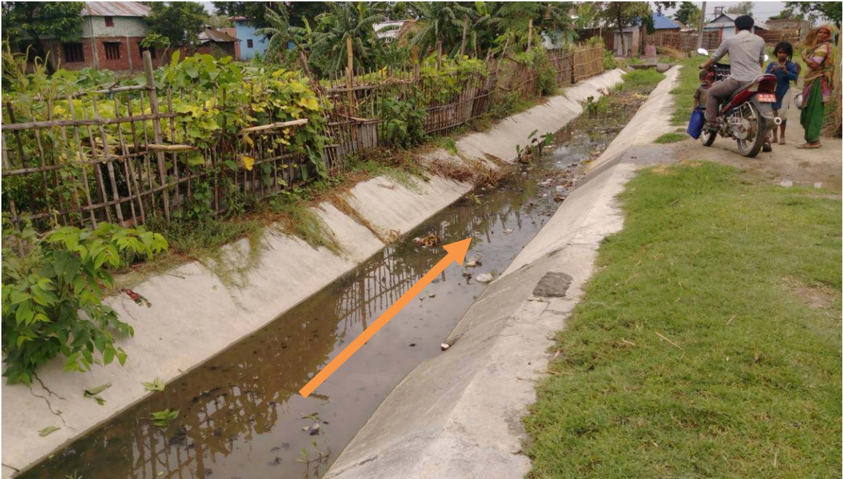
Pic.3:S10-T4, (Ch. 0+020), About 30 cm depth of silt deposited on 1.64
