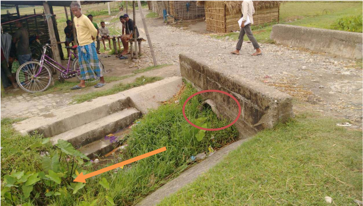
Pic.11: S10-T4, (Ch. 1+293), About 40 cm depth of silt deposited and vegetation growth at d/s side of PCV3 and spalling on pipe of PCV3 at d/s
