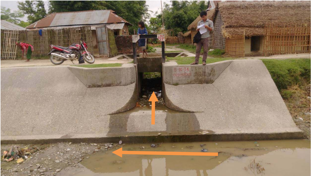
Pic.1: S10-T4, (Ch.0+000), Corrosion on bracing frame, Damaged gate plate of CV1
