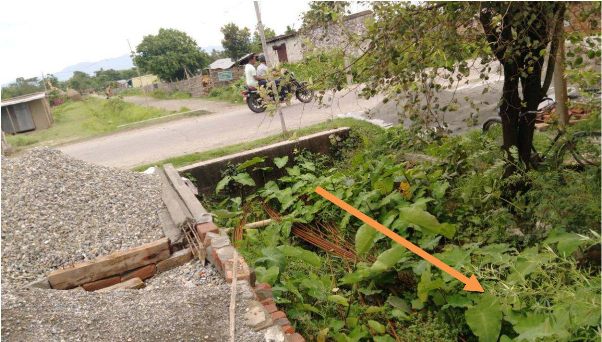
Pic.13: S10-T4, (Ch. 2+595), about 40 cm depth of silt deposited and vegetation growth at u/s and d/s side of PCV7
